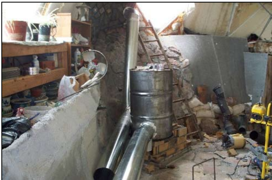
Fifty-five gallon drum installed with exhaust pipe being attached. The pipe exits the house just above ground level by the window.
