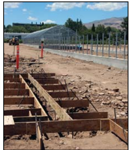
Hoop house construction has begun as part of the University of Nevada, Reno's High Desert Farming Initiative at the Valley Road Field Lab. Photo by Mike Wolterbeek, University of Nevada, Reno.
