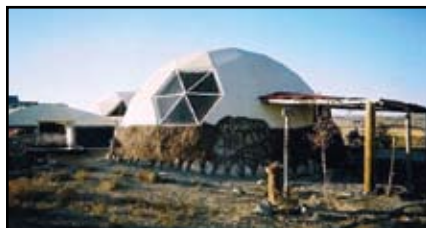
Rock wall going up around base of dome with cob concrete mixture covering earth bags.
