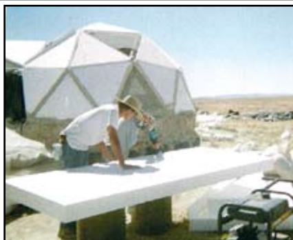
Above: Chad and Tami cut triangle panels out of the 4 x 8 sheets of five-inch foam. The bathroom dome is behind them showing the filled seams and the cob and rammed tire foundation.
