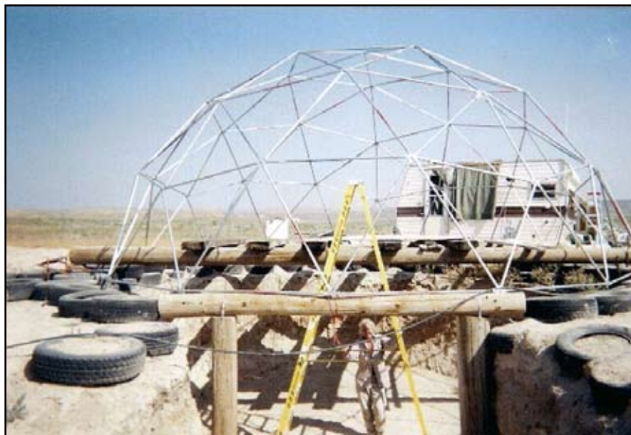
Tami stands with a 14-foot ladder in one of the bedroom domes. It is 20 feet from ground to top of dome.
